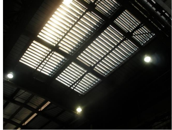
Light from a MatrixVent unit AFTER
